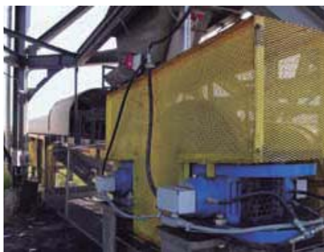
Twiflex VS180 spring-applied hydraulic released brake units fitted to an overland coal conveyor in West Virginia.
